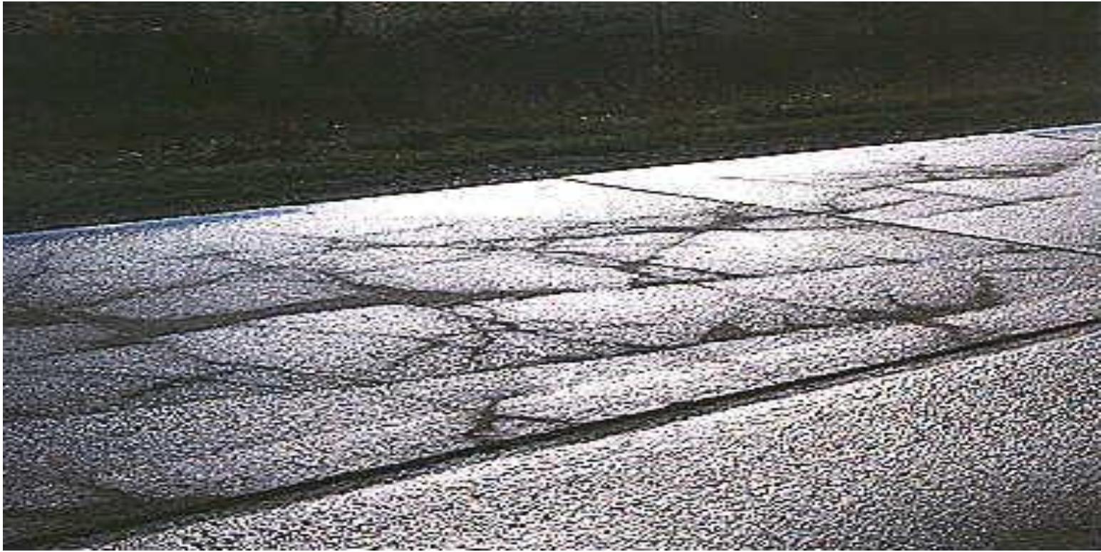
Cracking due to plastic shrinkage
