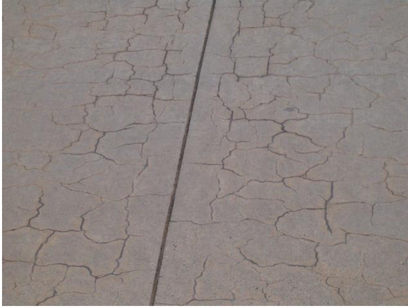
Airfield concrete subjected to AAR
