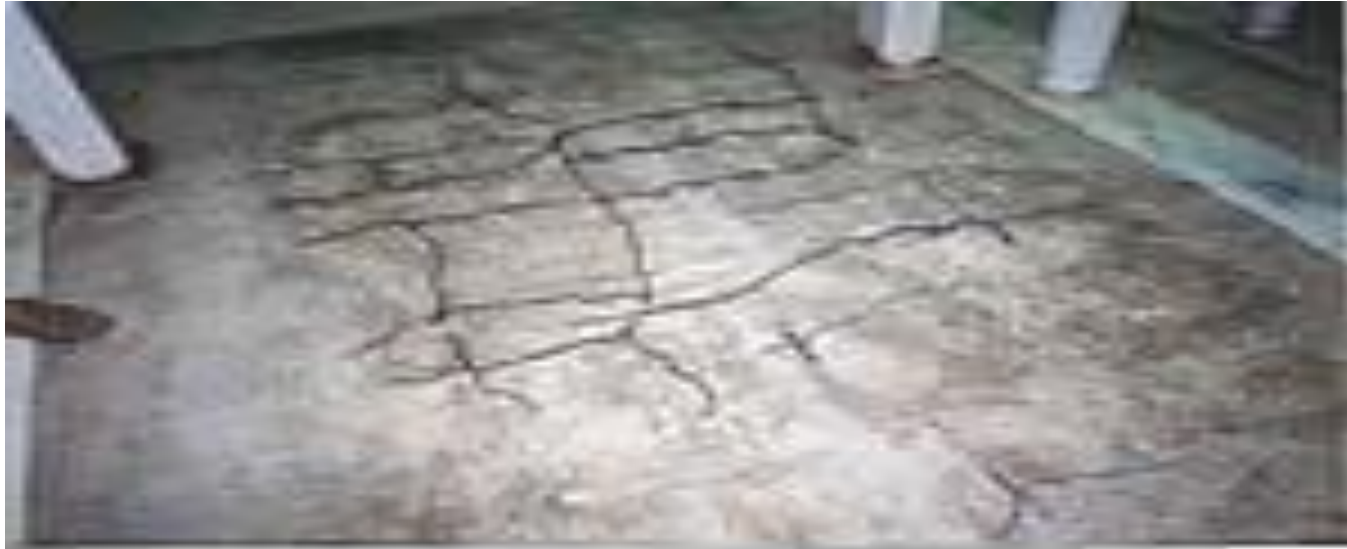
Cracking due to drying shrinkage
